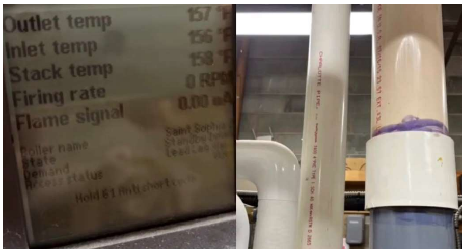
Figure 8: A 2-year-old high efficiency installation which has a stack temperature of 158°F and PVC venting, which can only tolerate temperatures up to 140°F. The PVC is beginning to show signs of failure via darkening.
