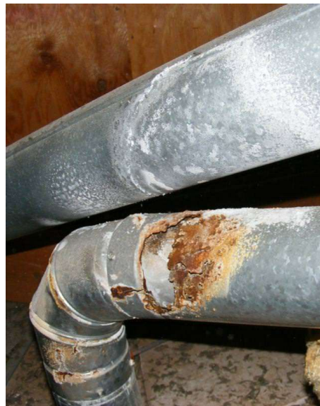
Figure 3: A B-vent that has been badly corroded by condensate (5).
