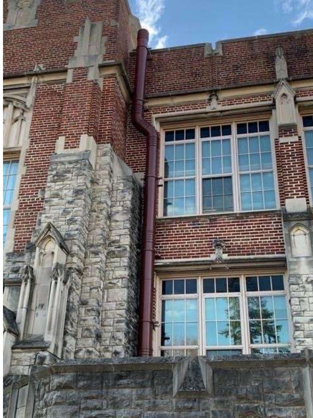
Figure 10: A tall vertical stack typical of a venting system.
