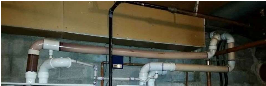
Figure 9: Unlisted PVC used for venting which has baked and turned dark due to high stack temperatures.
